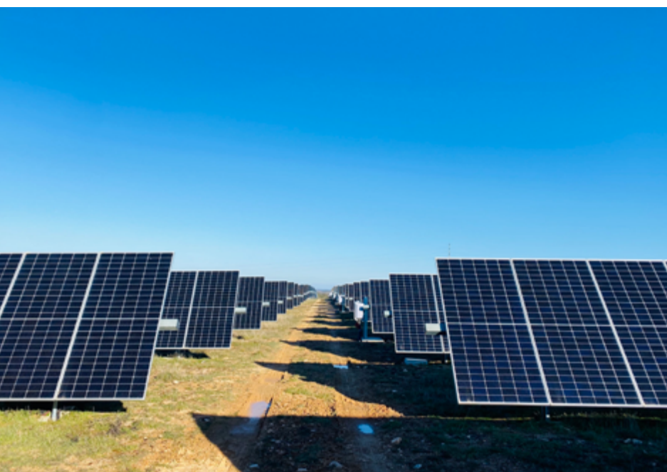
Plant " Betty" with tracker modules
