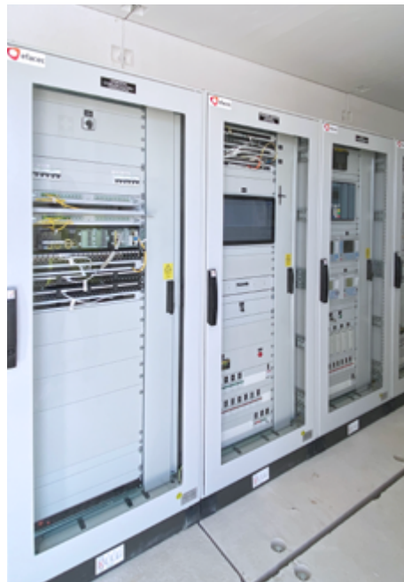
Collection and processing of all data in the E-house
